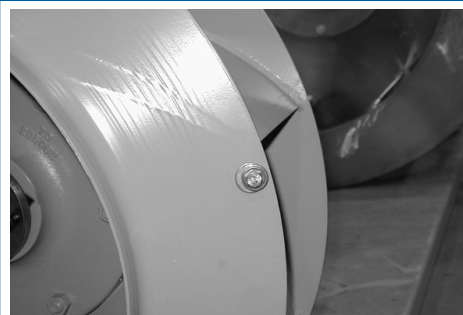
Permanently secured stainless steel bolts, nuts and washers used as balancing weights after paint
