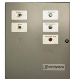
Typical Industrial Remote Panel
