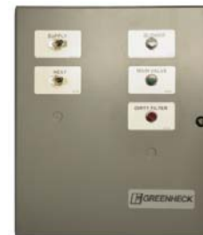
Typical Industrial Remote Panel
