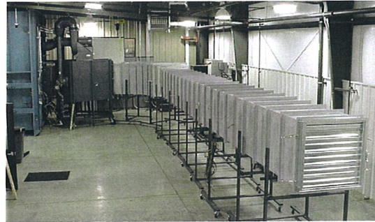
Greenheck expedited the testing process by simulating heated air flow during fire emergencies in its UL Certified on-site testing lab.
