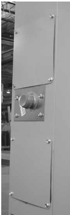
Distributor Access Panel
