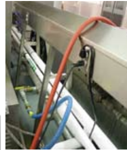
Figure 3 (left) and 4 (below) show an attempt at a field-built utility distribution system compared to a well manufactured, pre-engineered system.
